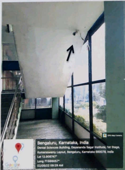
CCTV camera at the entrance of Dental College
